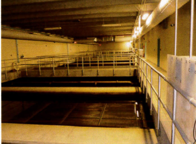
Upflow Clarifiers and Filters
